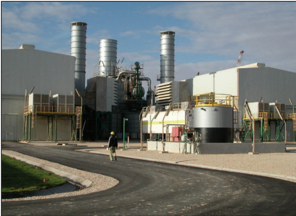
■ The Mellitah Gas Compression Station owned by GreenStream on the Libyan coastline at the head of the 323 mile (520 km) 32 inch (81 cm) sealine exporting Libyan natural gas to Italy.
