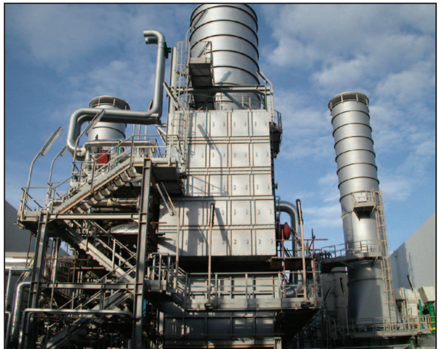
■ Detail of the HRSG producing steam for the adjacent gas processing plant.
