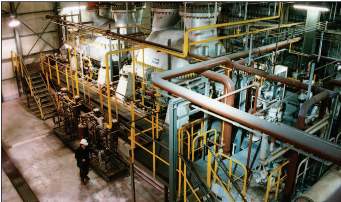
■ Low BTU fuel gas compressors driven after a 100 MW generator by a Frame 9E gas turbine at the Ilva steel mill in Taranto, Italy. Three similar units are installed in this steel mill.
