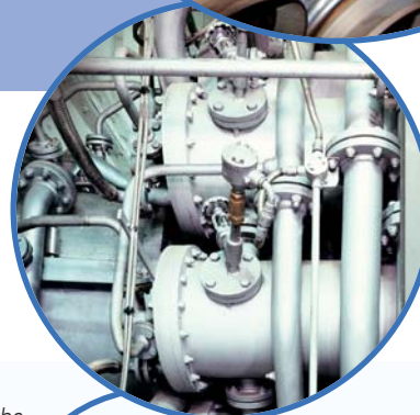
External view of the DLN combustion chamber
