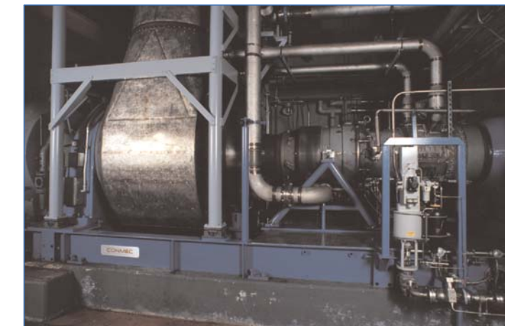
GE's Conmec installation with an AVON gas generator retrofit and an upgraded RT-48 power turbine
