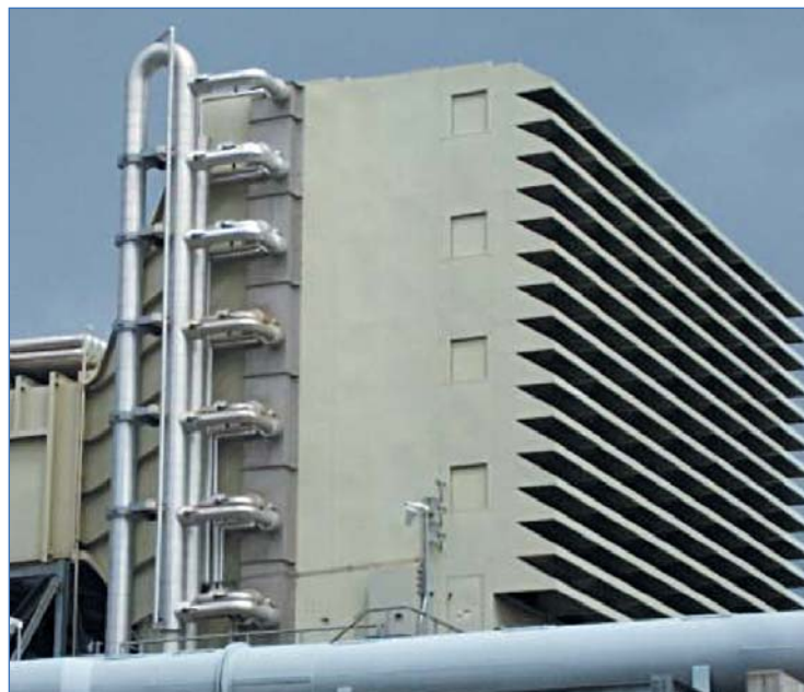
Example of chilling installation
