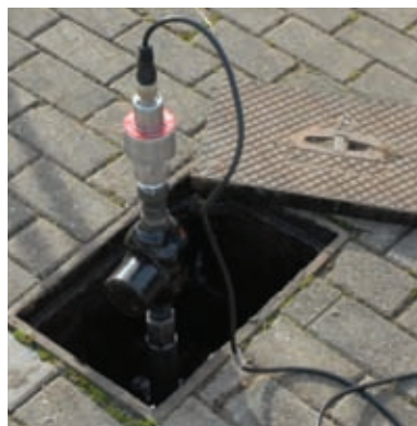
Hydrophones are installed at various intervals along the pipeline and can be easily removed or repositioned at any time.
