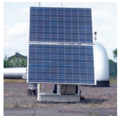
Solar panels can be installed to provide all necessary power, making ThreatScan a truly self-contained solution.
